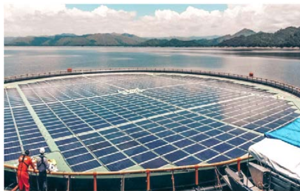
Dezhou Dingzhuang Floating Solar Farm
