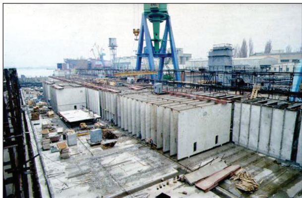
Fig. 1. Formation of the steel-concrete pontoon of the floating dock with the buoyant power of 25,000 t in the docking chamber of the plant
