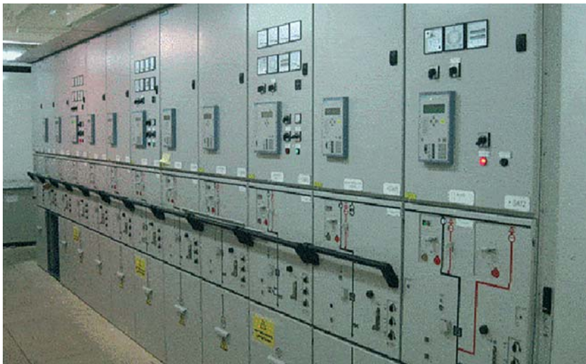
Figure 11.3 – The main switchboard device [21]
