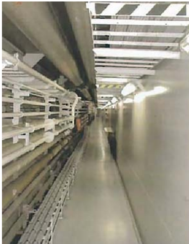
Figure 11.2 – Cable trays and pipes in the corridor between the forward and aft engine room of a stone dumping vessel [21]
