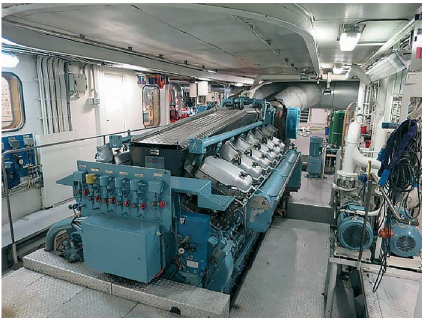
Figure 10.1 – Engine room of the ferry ship [28]
