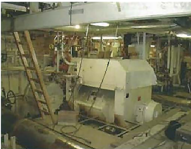
Figure 11.1 – Main-engine driven generator [21]
